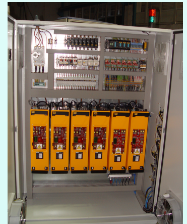
Main Electrical Cabinet
