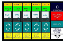
Operating Touch Screen Panel
